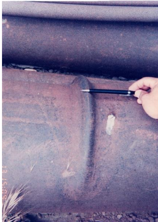
Figure 87: Example of Local Pipe Wall Buckling
