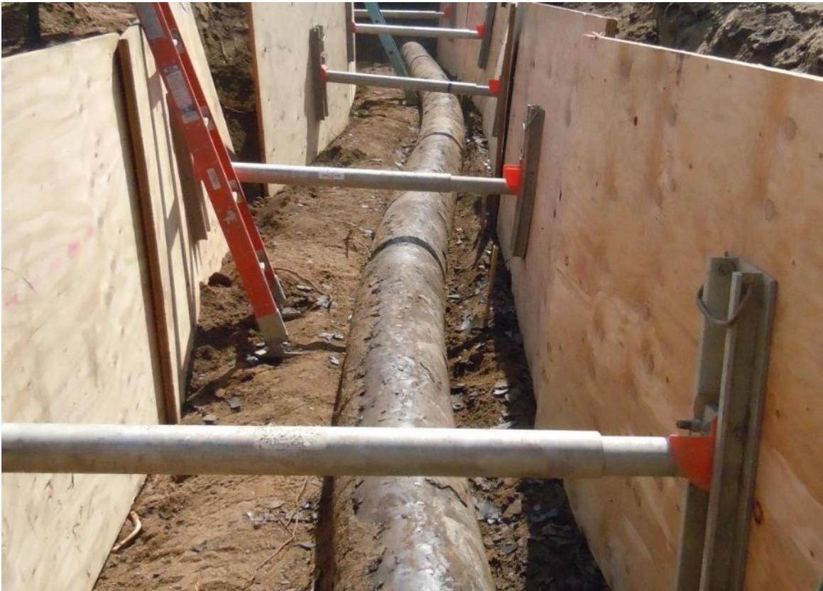
Figure 93 Deformed Shape of Exposed NPS 12 Pipeline at the San Andreas Fault Crossing
